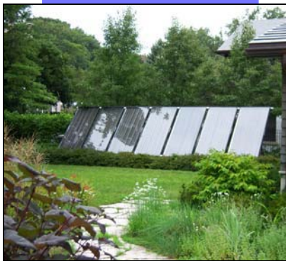
Several 4'x8' hot water solar collectors installed along the driveway provide much of the heat for the radiant-floor heating system.
